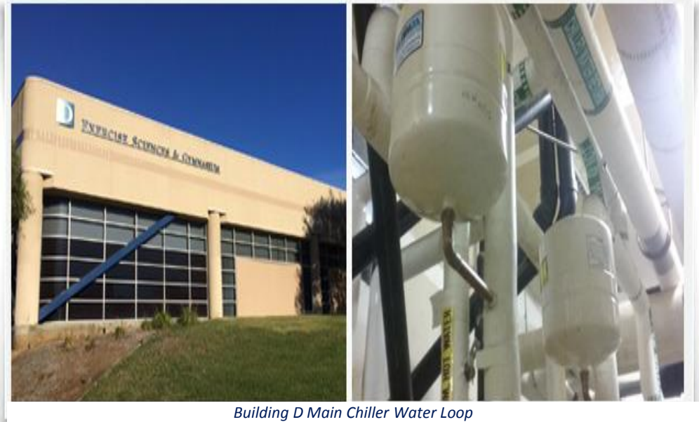
Building D Main Chiller Water Loop
